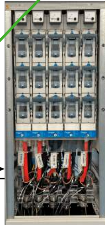
Electrical distributor in the low-voltage grid ( grid level 7)
